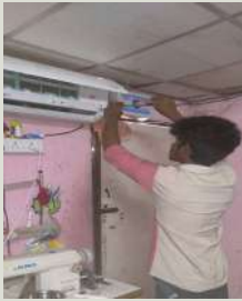
Lispan J Electrical&AC Wiring New Tech Services AC Technician Salary:10,000
