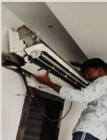
Balaji P Electrical&AC Wiring Everest Air Conditioner Sales & Services Electrician Salary:12,000
