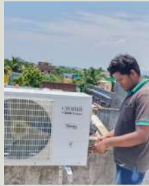
Nirmalraj L Electrical&AC Wiring Croma Sales & Services AC Technician Salary:10,000
